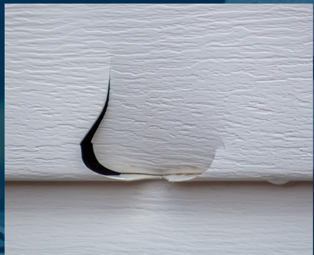
2. Cracking/physical performance loss: Moisture | Temperature cycling | Mechanical stress
